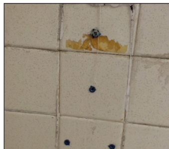
NO MORE DISPENSERS RIPPED OFF THE WALL
